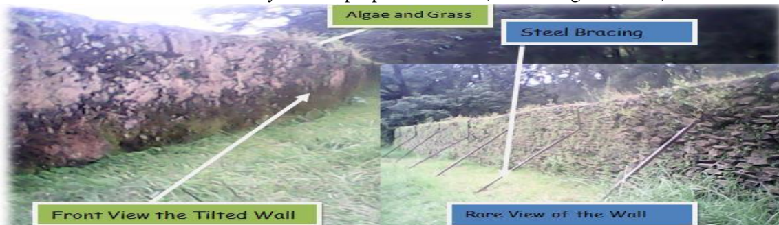
Figure 10: Leaning Of the Masonry Wall in the Royal Palace Near to the Main Road
