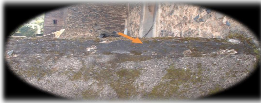
Figure 7: Mortar deterioration due to Chemical Reaction
