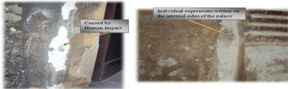
Figure 9: Mortar deterioration due to Mechanical action
