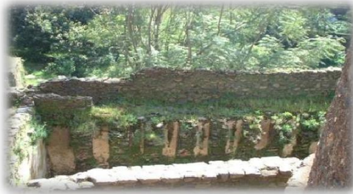
Figure 1: Buildings in deplorable state
