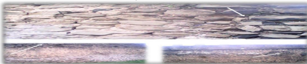
Figure 11: Mortar re-pointing in the internal and external appearance of the palace wall
