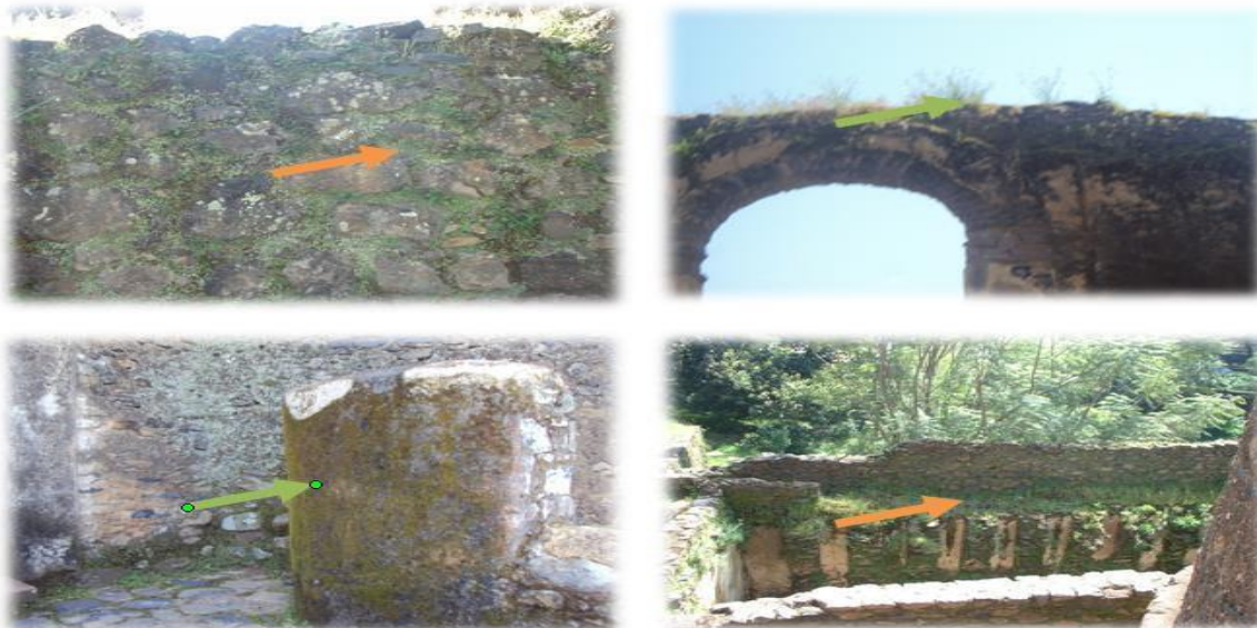
Figure 8: Mortar deterioration due to Biological Causes
