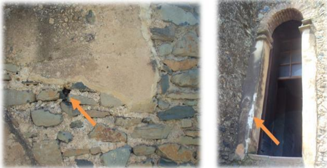
Figure 6: Deterioration of rendering Mortar
