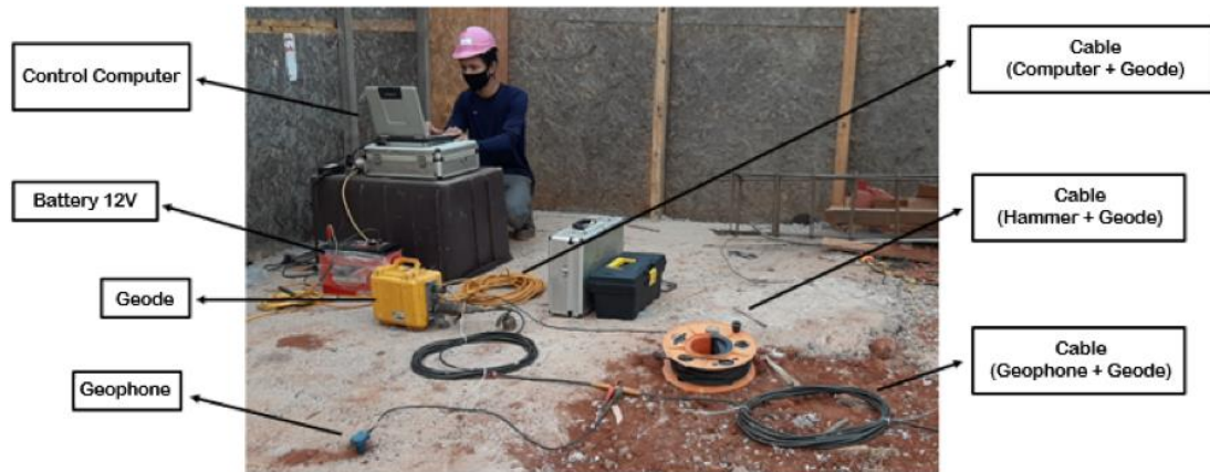
Figure 3. The identification of each equipment is indicated in the rectangles. The installation site is located inside the construction site.
