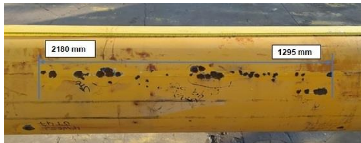
Figure 8. Corrosion mapping inspection: a) PIG going through the tube, b) Corrosion expected to be found.
