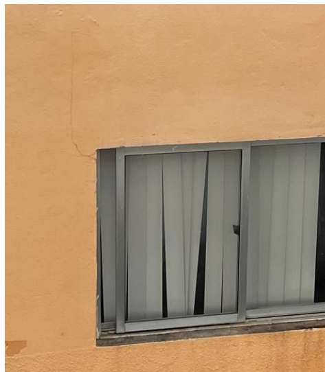
Figure 29. Vertical crack on the posterior face of Block G
