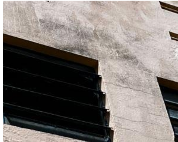
Figure 2. Dirt on the top of a window of the front facade of block G
