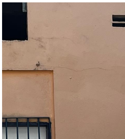
Figure 27. Horizontal cracks at gap ends on the rear facade of block G
