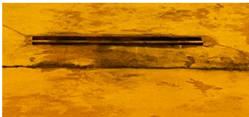
Figure 14. 45° crack in opening in the right side facade of block G
