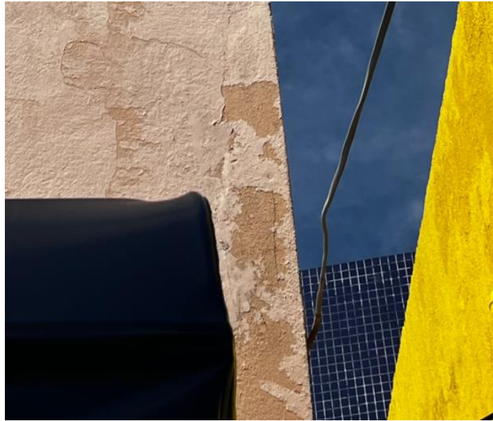
Figure 5. Paint detachment on the abutment
