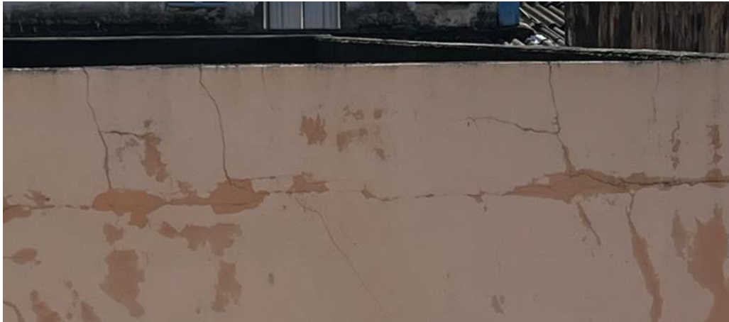
Figure 28. Vertical and horizontal cracks on the back facade of block G
