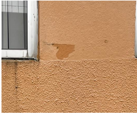
Figure 25. Paintwork detachment on the posterior facade of block G
