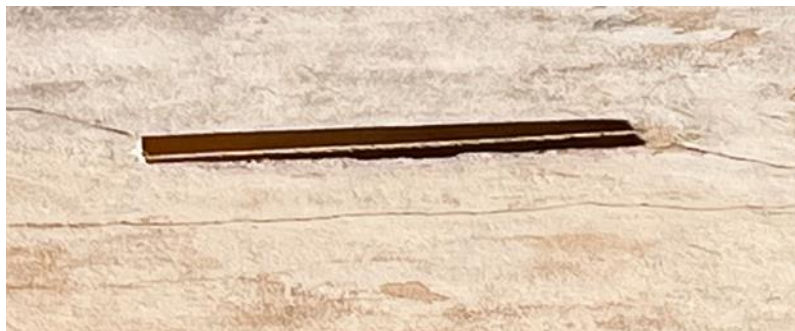
Figure 21. 45° crack in the left lateral facade of block G
