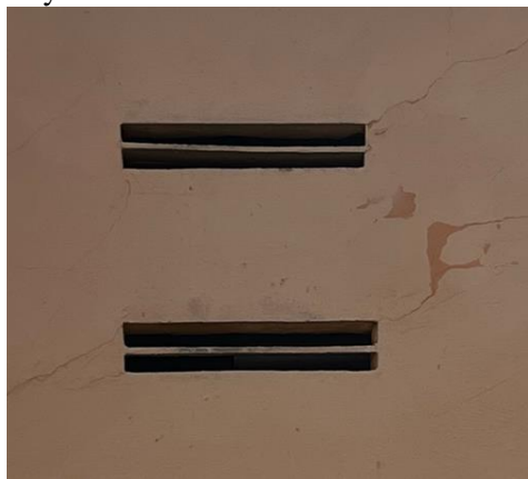
Figure 26. 45° crack in the rear facade of block G
