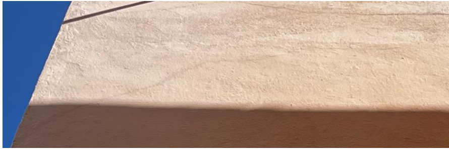
Figure 20. Cracks in the upper part of the left lateral facade of block G
