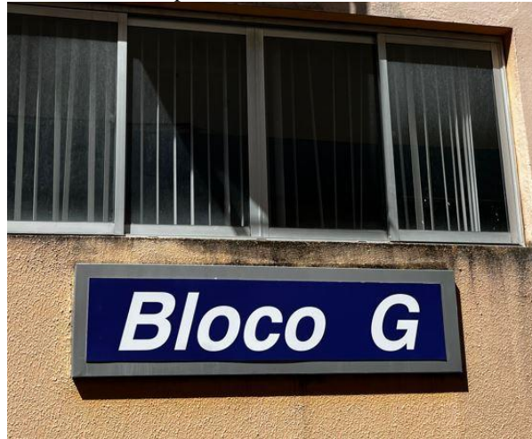
Figure 3. Dirt between plate and window of the front facade of block G
