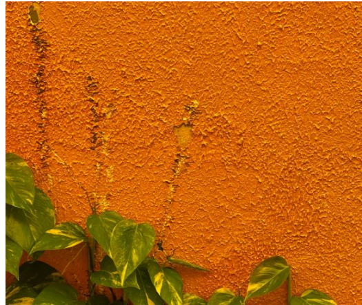
Figure 12. Paint detachment on the base
