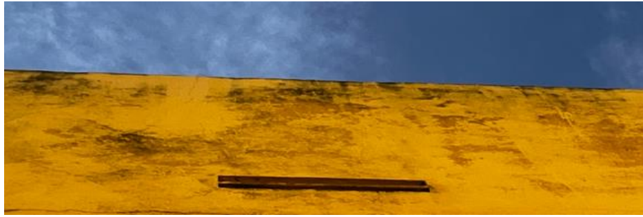
Figure 9. Dirt on the upper part of the right side facade of block G
